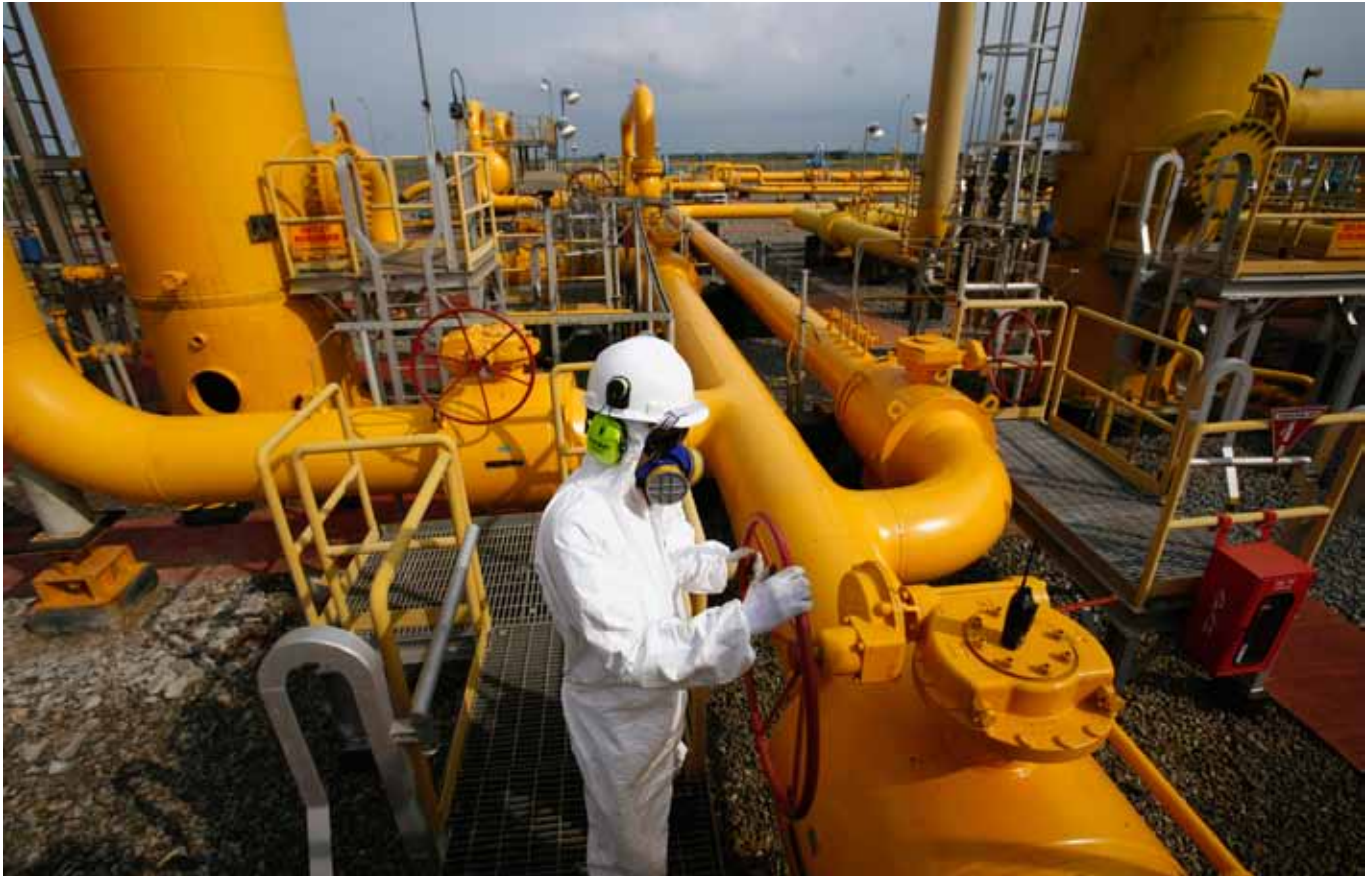
A PT Perusahaan Gas Negara Tbk (PGN) employee checks pipes at a gas receiving-and-transmitting station in Bojonegara, Banten province, Indonesia. REUTERS/Supri
