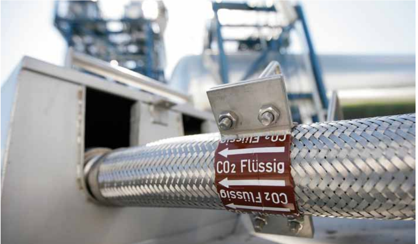
A flexible tube for CO 2 is pictured in Spremberg, Germany, as part of Vattenfall's CO 2 -free power plant. This is part of a pilot project for carbon capture and storage (CCS) – the first plant in the world that will take toxic emissions from coal and bury them in the ground. REUTERS/Hannibal Hanschke
